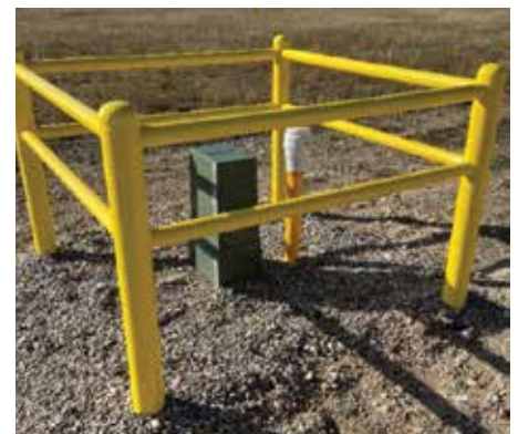
Above grade enclosures of AC mitigation PCR and RMU
