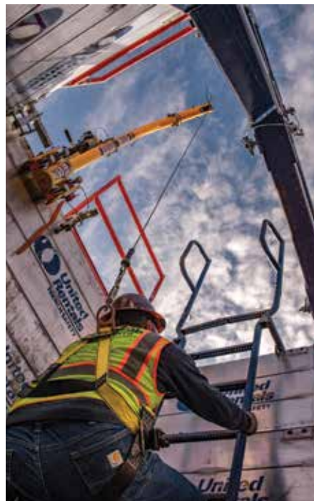
MAPS with fall protection, ladder and guard rail
